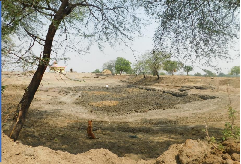
Photograph of after completion of Work at Site-3 (Dihili tank), Village Name- Gandharla
