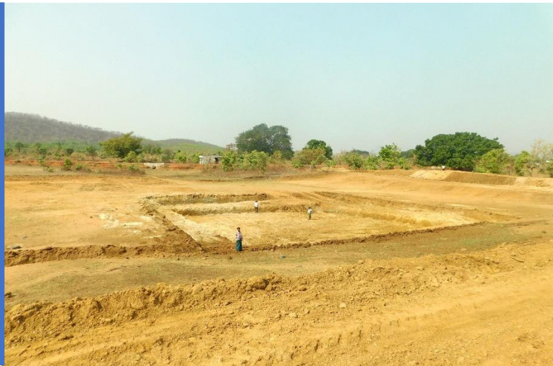
Photograph of After Completion of Work at Site-1 (Khinbasa tank), Village Name- Batharla
