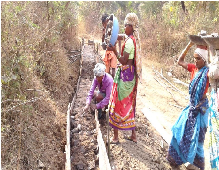
Construction of Guard wall near newly constructed WHS (site 2 -Sundhimunda Village , Malmuda tank)
