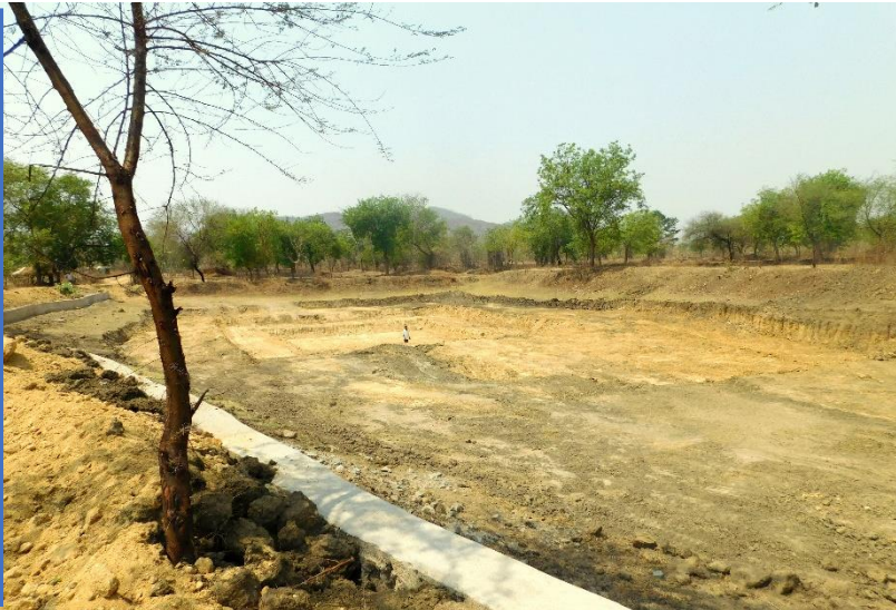
Photograph of after completion of Work at Site-2 (Malmunda tank), Village Name- Sundhimunda, malpada
